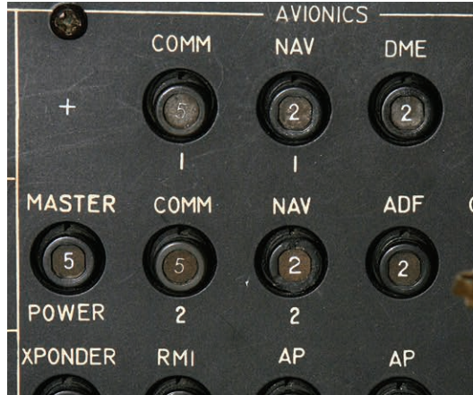
Figure 11-5-14. Circuit breaker panel arrangement.
