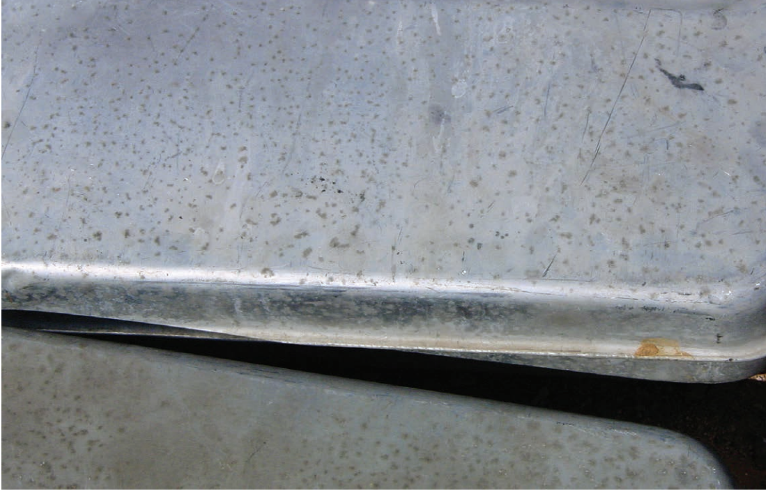
Figure 7-2-1. An example of uniform surface corrosion.
