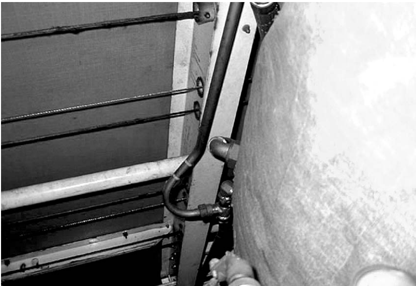
Figure 9-8-12. The area below the floorboards around galleys and lavatories is a likely site for corrosion. The large object on the right is a potable water tank, with a main floor beam running vertically in this picture.
