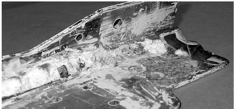
Figure 9-8-9. This casting developed extensive corrosion when the built-up sealant cracked and allowed water to contact the metal. The part appeared sound until corrosion extended beyond the sealant.
