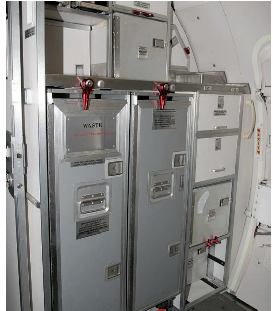
Figure 9-8-11. Exposure to water and food items makes galley areas especially prone to corrosion.
