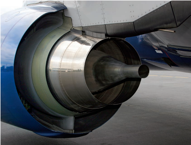
Figure 9-8-10. Exposure to high heat and corrosive exhaust gases make engine exhaust areas susceptible to corrosion.
