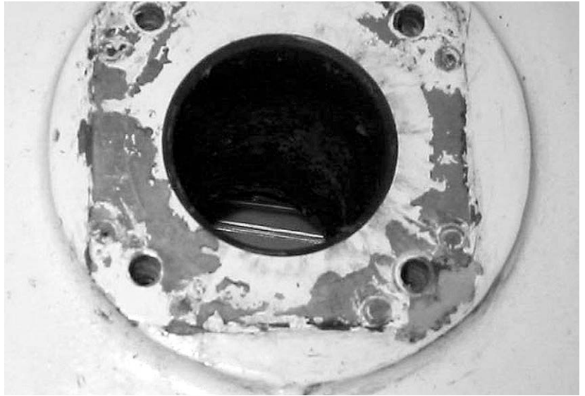
Figure 9-8-2. This magnesium casting was installed in a passenger door. Pitting corrosion formed on the lower edge of the gasket (removed) when the sealant became worn. The pitting is more than 0.1 inch deep.
