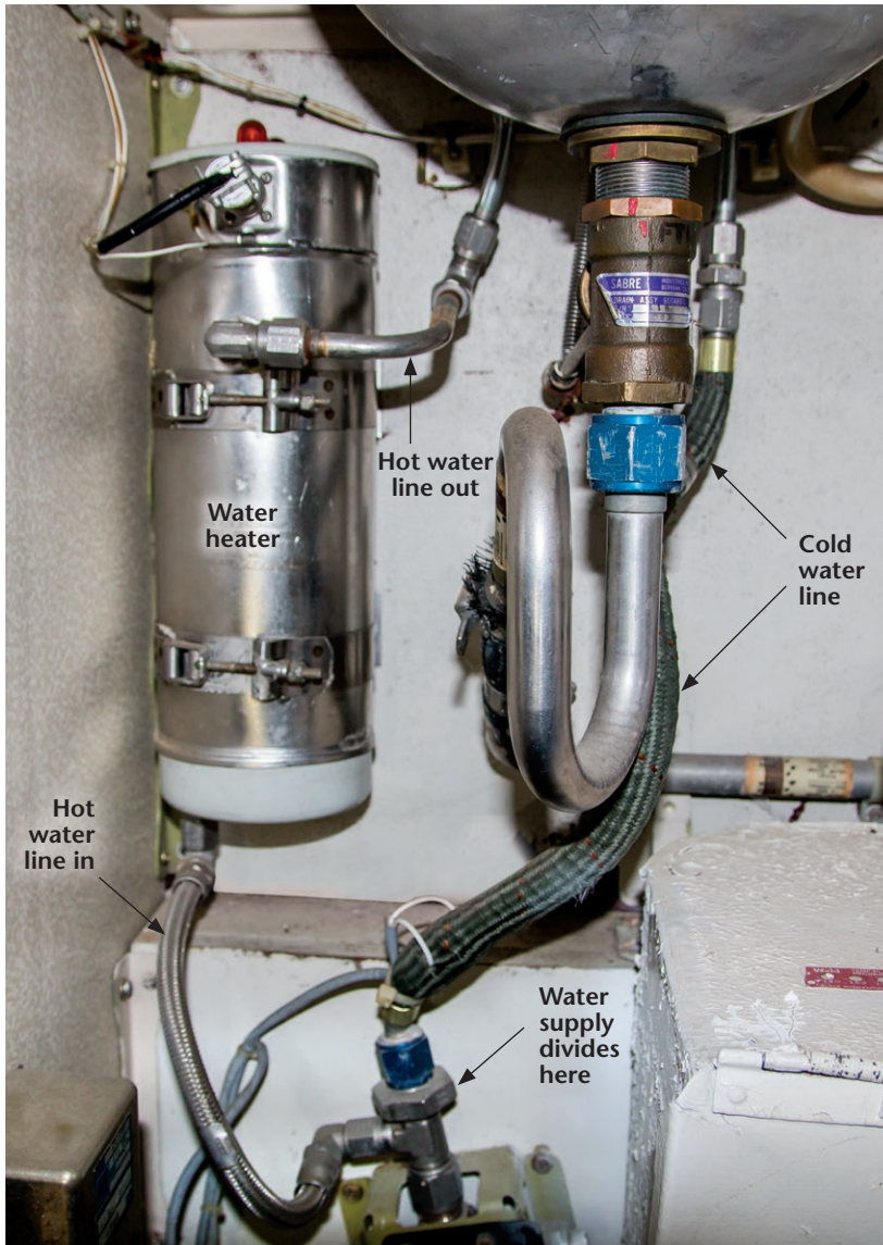
Figure 2. Under the lavatory sink, the lines lead to the cold faucet and to the hot faucet via the water heater.
