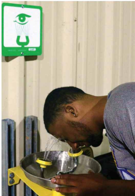
Figure 6-2-2. An OSHA-approved eyewash station is required and extremely important!
