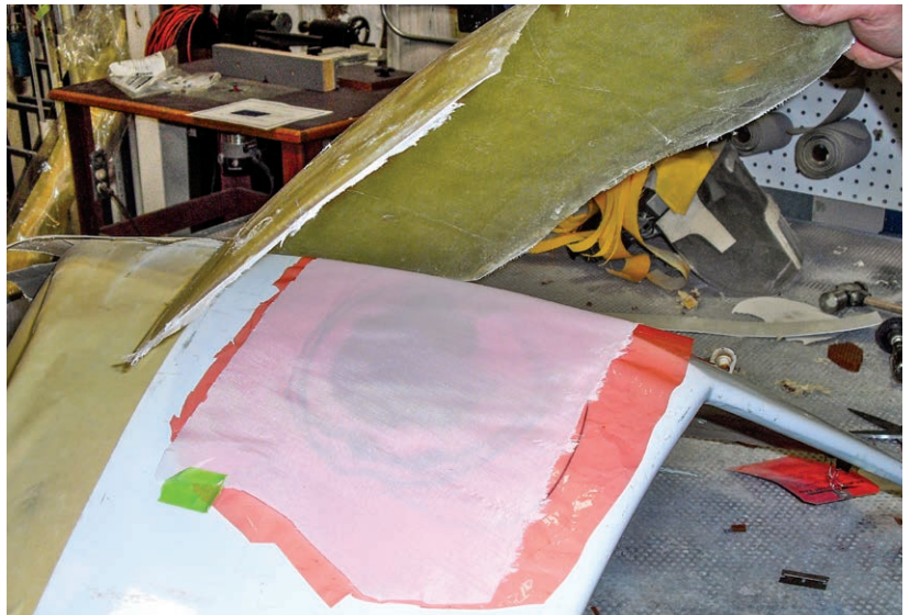
Figure 12-7-11. The splash mold is laid over the repair area and taped down temporarily until the vacuum is applied to hold it in place during the cure.
