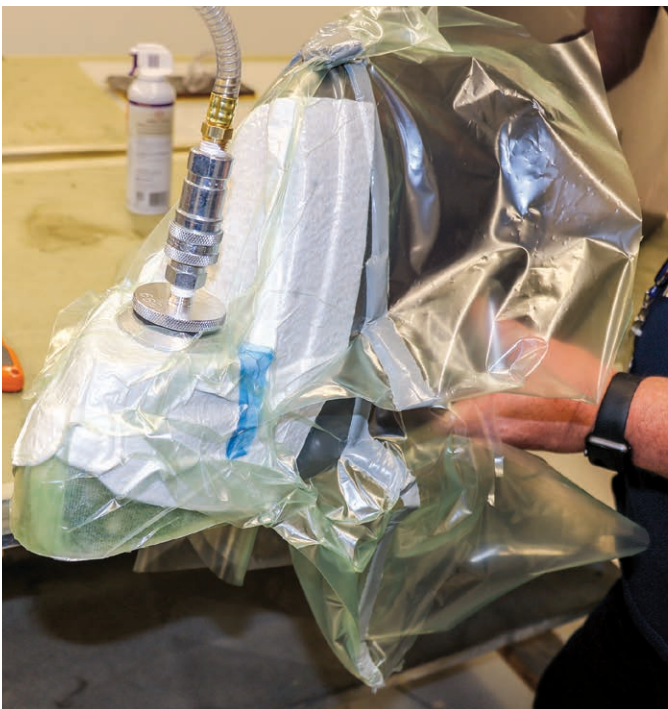
Figure 7-5-2. The part is bagged on the inside and outside with sealant tape and bagging film. The top bagging film is brought over the top of the repair and sealed to the bagging film attached to the inside of the part.
