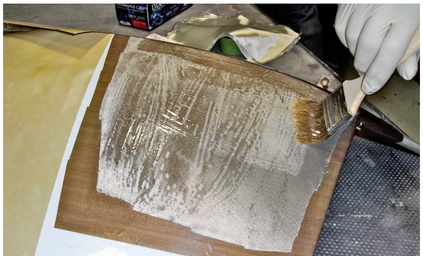
Figure 12-7-7. Build up the mold by layering fiberglass with resins. In this example, five layers of fiberglass were used to build up the mold.
