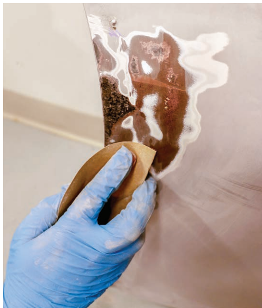
11-5-1. Remove the paint from the part, being careful not to damage the structural layers.
