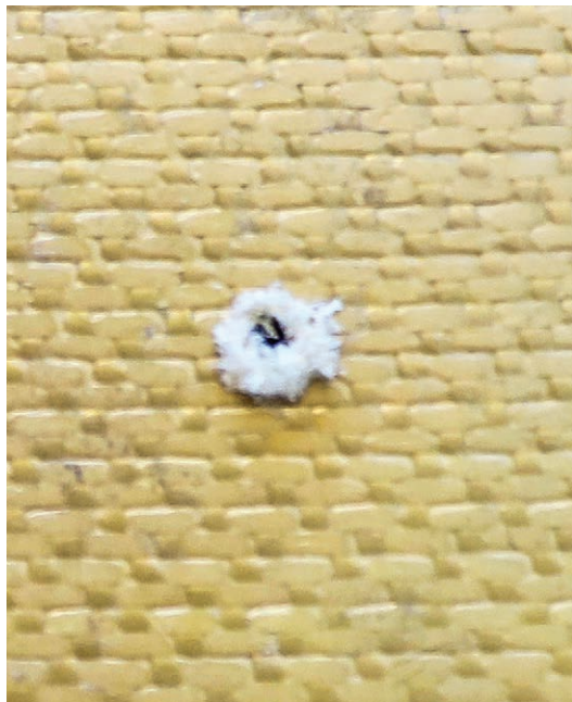
Figure 9-2-2. The fuzzing around the hole is caused by the drill pulling the fibers and then cutting them with a traditional sheet metal drill.
