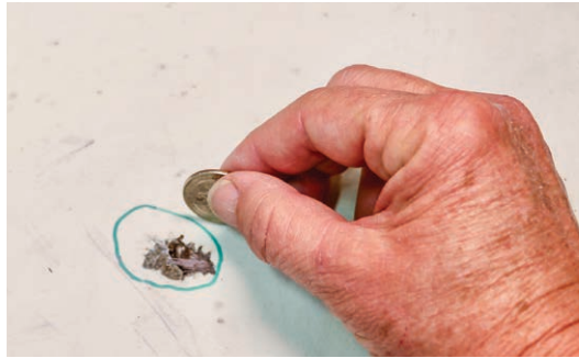
Figure 11-3-1. Coin tapping a part around areas suspected of delamination. The circled area is larger than the hole because delamination was detected.
