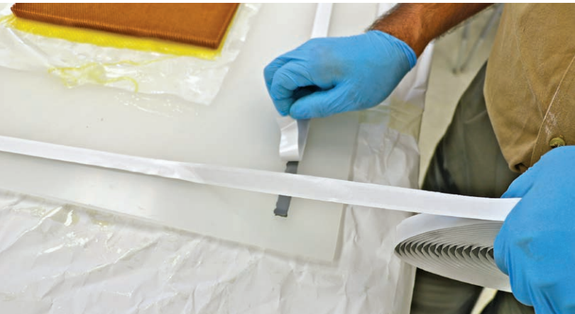
Figure 7-2-6. Applying sealant tape around the repair area. Overlap the ends to seal all air leaks.
