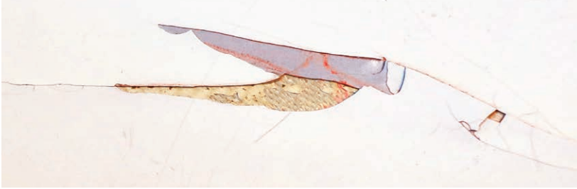
Figure 11-2-3. Areas that show cracks should be inspected more thoroughly to see if the cracks are only in the paint or have propagated into the fiber materials.
