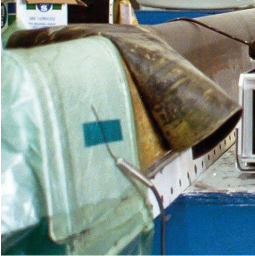
Figure 12-7-4. The repair is vacuum bagged and cured, then the boot is reinstalled.
