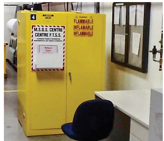
Figure 10-1-4. Storage locker marked Flammable for resins, catalysts, and solvents. SDS and certifications should be stored next to the locker.
