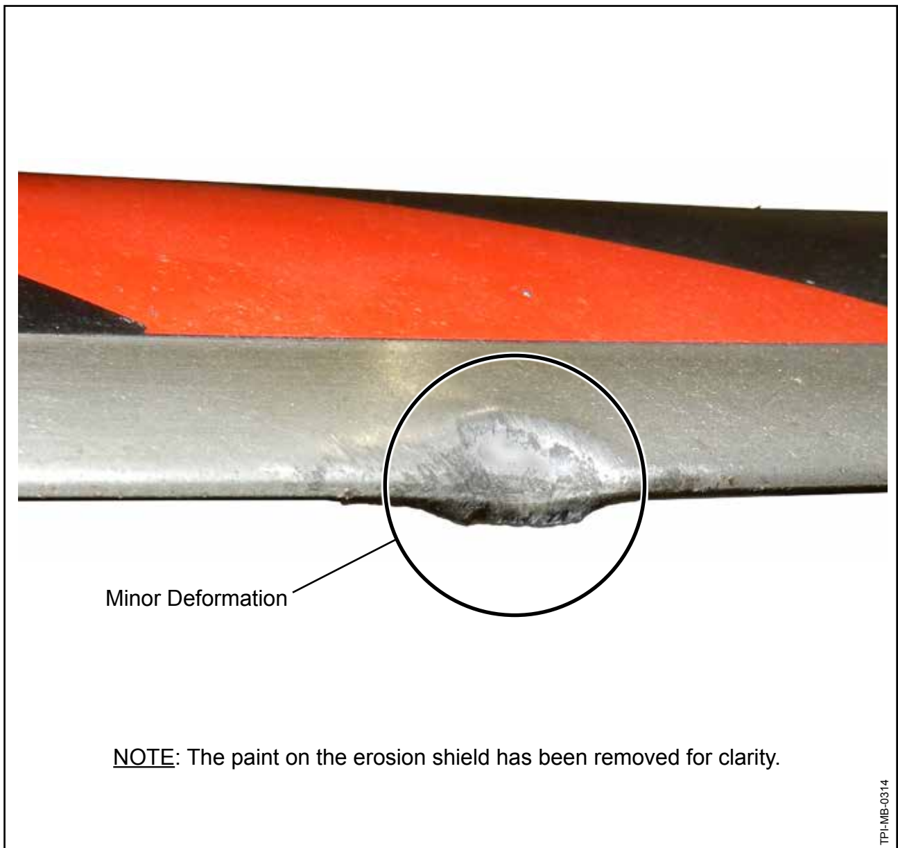
Erosion Shield: Minor Deformation Figure 2-1
