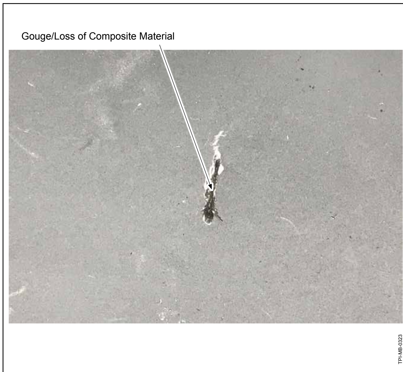
Blade Surfaces (except the Erosion Shield): Gouge or Loss of Composite Material Figure 2-6
